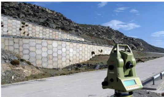
Automatic surveying system (ATS)
