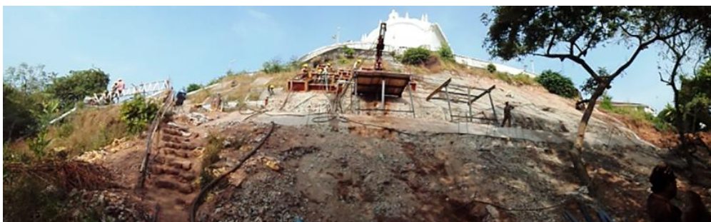
In-place inclinometers and piezometers installed for online slope monitoring at Cabo Fort, India
