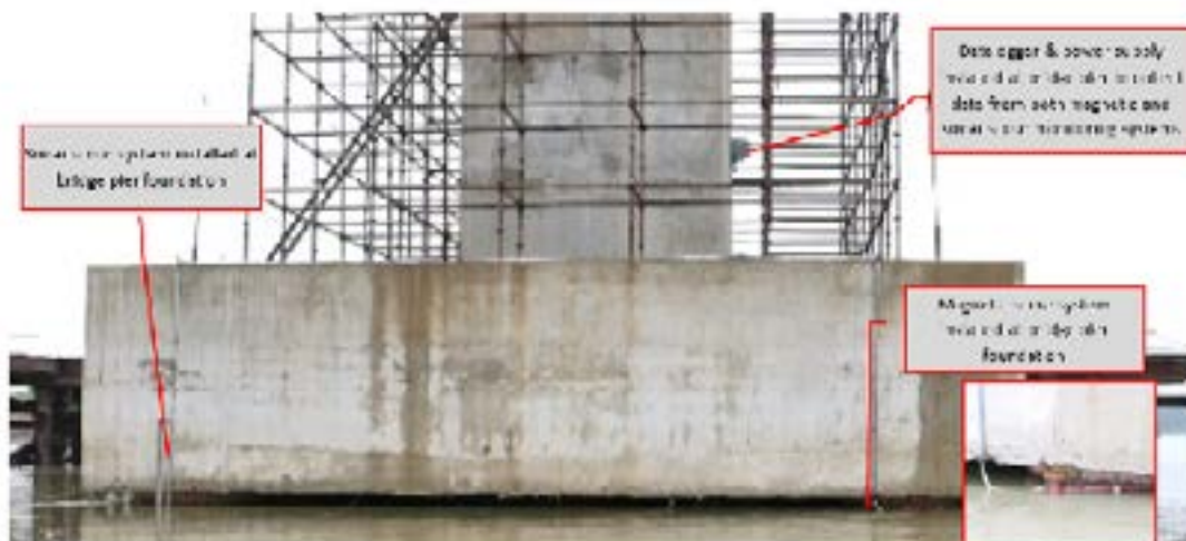
Scour monitoring system (magnetic and sonar with datalogger) installed at a bridge in India
