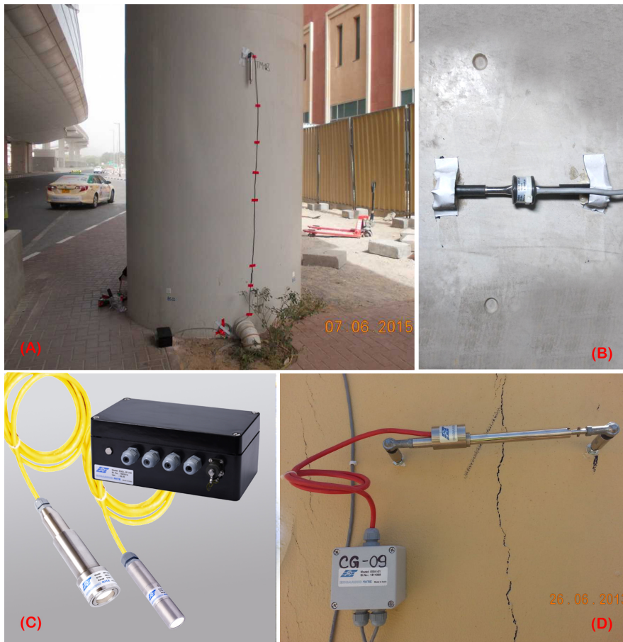
FIGURE 4: SHOWS TYPICAL LOW POWER SENSORS DEPLOYED FOR MONITORING CIVIL ENGINEERING STRUCTURES. PICTURE A – SENSITIVE BIAxIAL TILT SENSOR MONITORING A BRIDGE PIER SUSPECTED OF DEVELOPING A TILT. BLACK BOX NEAR THE BASE CONTAINS A BATTERY POWERED DATA LOGGER WITH CELLULAR NETWORK CONNECTIVITY. THIS IS AN EXAMPLE OF AN USER MONITORING ISOLATED PROBLEM AREAS SPREAD OVER A LARGE AREA WITH A FEW AUTONOMOUS SENSORS TOGETHER WITH CLOUD SERVICES. PICTURE B – STRAIN GAUGE FOR MONITORING STRESS ON A STRUCTURE. PICTURE C –WATER LEVEL/ PIEZOMETRIC PRESSURE SENSORS TO MONITOR WATER LEVEL IN A RIVER OR PIEZOMETRIC PRESSURE IN THE GROUND. PICTURE D – CRACK METER MONITORING A CRACK IN A STRUCTURE THAT HAS STARTED SHOWING SIGNS OF MOVEMENT.
