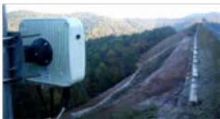
GATEWAY INSTALLED FOR WIRELESS MONITORING
