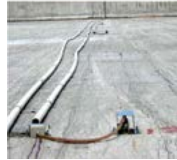
TILT METER INSTALLED AT CONCRETE FACE OF DHAULIGANGA CFRD,INDIA
