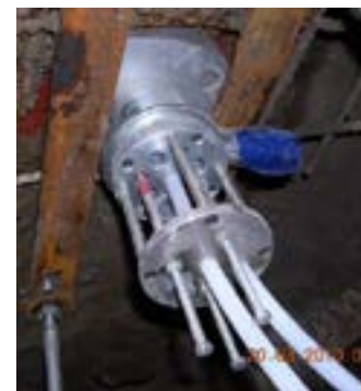
Load cell & BHE in powerhouse at Koprubasi HEP, Turkey
