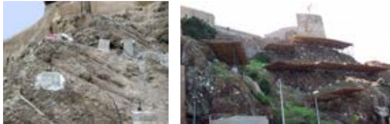
Borehole extensometers and in-place inclinometers installed for online slope monitoring at Al Mirani Fort, Oman
